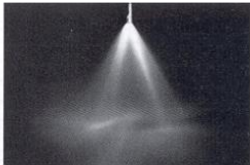
Distorted spray from damaged or clogged nozzle
